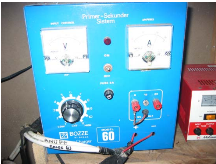
Figure 3: Electrical: supply 12V, 20 Amps total for all biorocks
